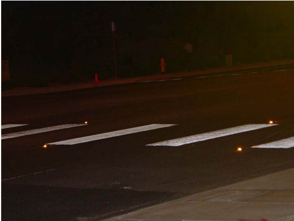
FIGURE 3 Installed in-pavement flashing light system at the study location
